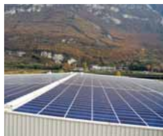
Industrial building CH Built in 2008 Power 48 kWp
