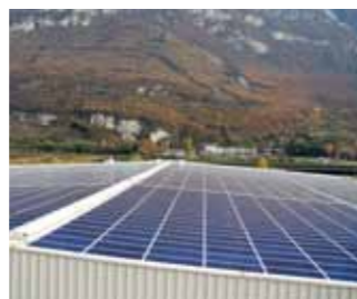
Industrial building CH Built in 2008 Power 48 kWp
