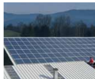
Agricultural building D Built in 2008 Power 20 kWp
